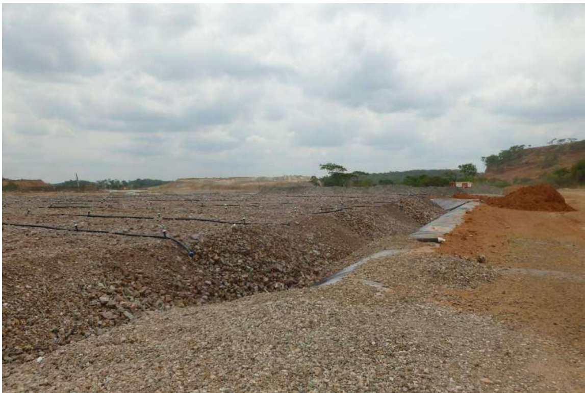
Figure 13-2 Heap Leach Pad
