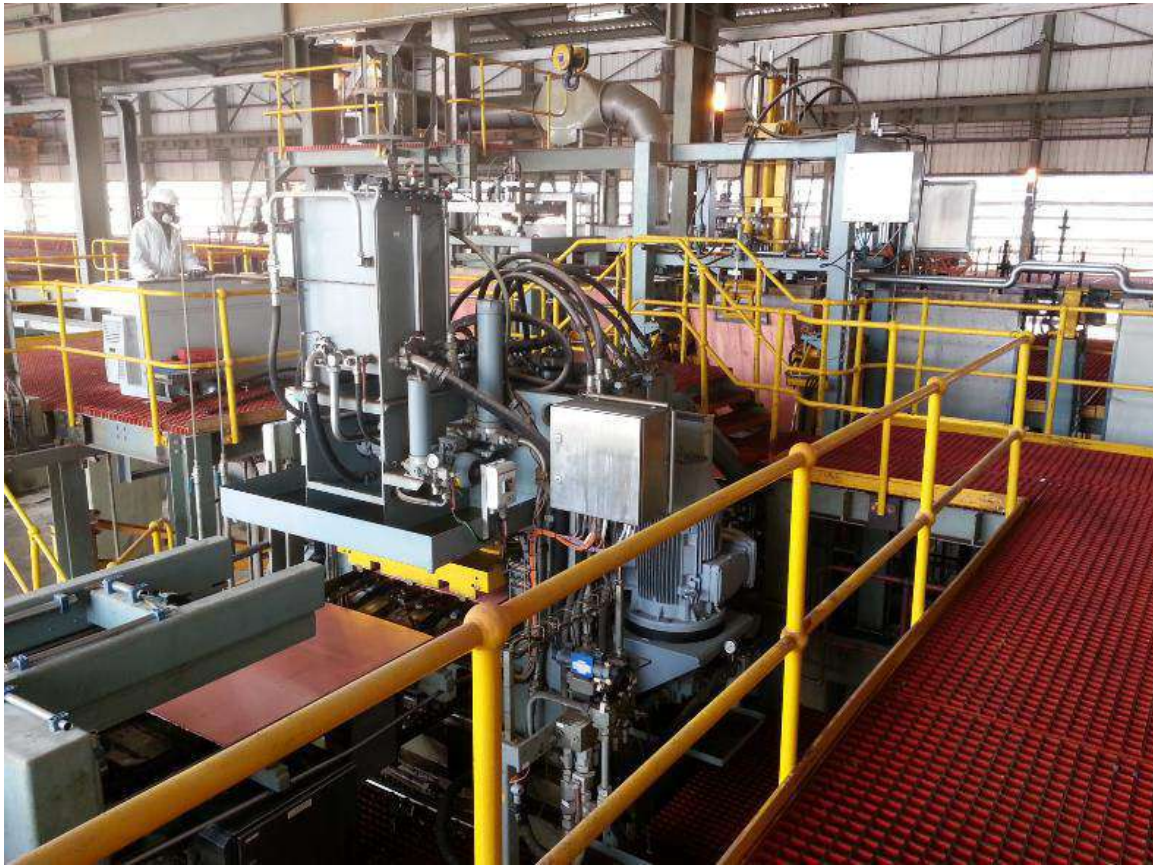
Figure 17-4 New Automated Stripping Machine (November 2013 Site Visit)
