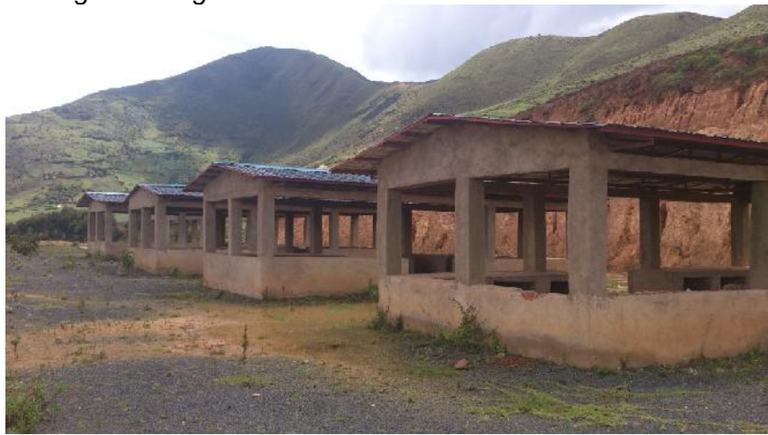
Marché du village CINJIRA non fonctionnel (construction non participative) - Twangiza Mining – Banro – Cinjira – Sud Kivu
