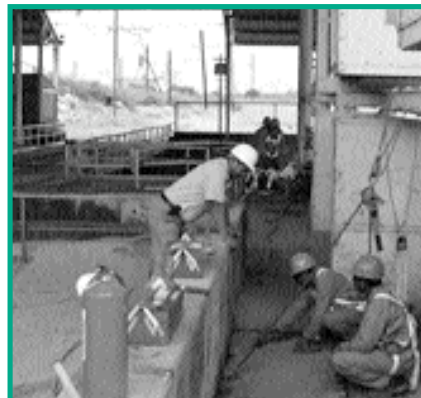
(left) A refurbished thickener in the concentrate receiving area of Luilu
