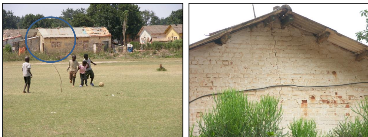
Picture 28: Football pitch and crack in houses in Musonoi
